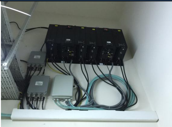
RU mounted on the road tunnel wall
