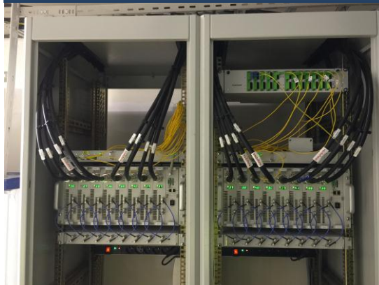
ACU & OCU installed in equipment room
