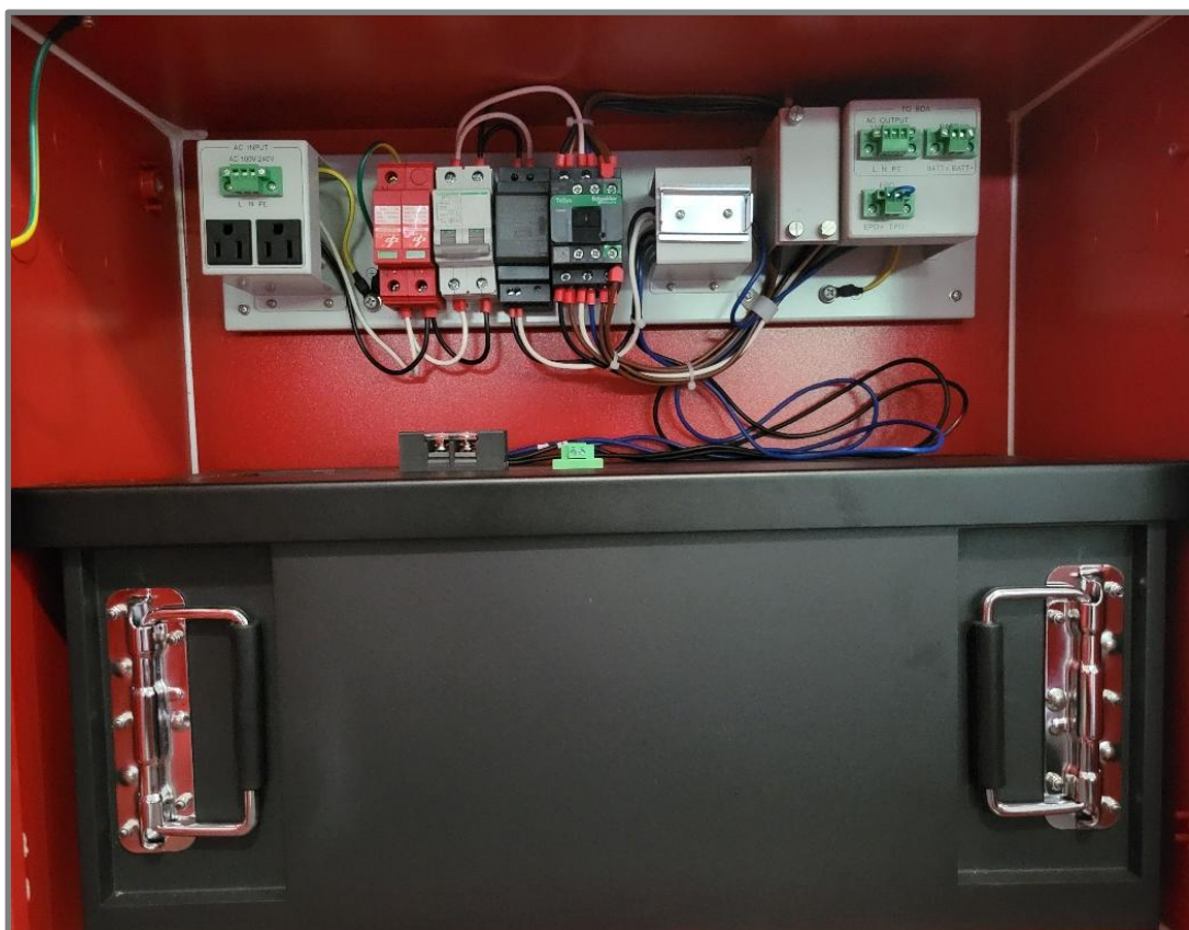
Figure 39: Battery Installation and Retaining Bracket
